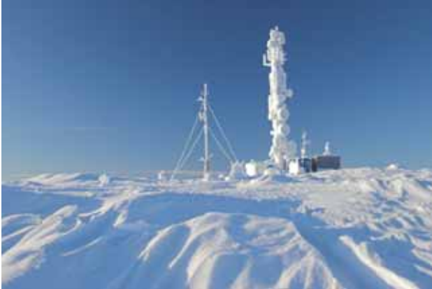
Cellular phone station.
